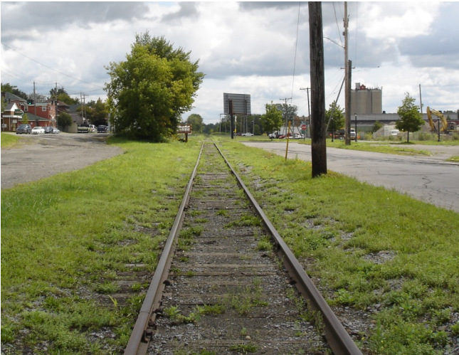
Existing railroad infrastructure running parallel to East Dominick Street and Railroad Street.
